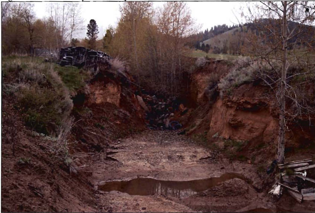
Photo by Kevin Bradford. A dam of broken concrete rubble, and tires wired together and staked down, has filled the gully half full and abated the force of the stream.
